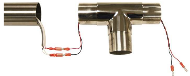
Figure C. Run supplied jumper wires between all fittings, including tees, elbows and 3-way corners. Adjustable fittings and dovetails should already have jumpers installed for your convenience.
